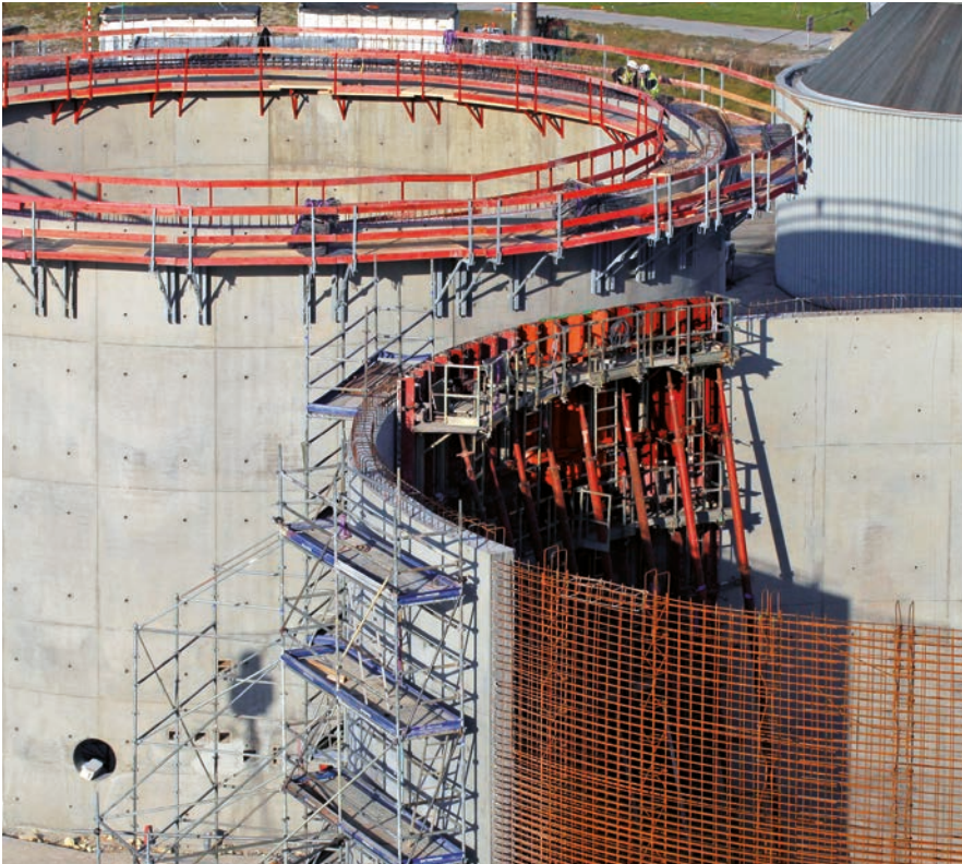
Waste water treatment plant, F-Brive la Gaillarde; Vigier/Sogea Sud Ouest, F-Toulouse
