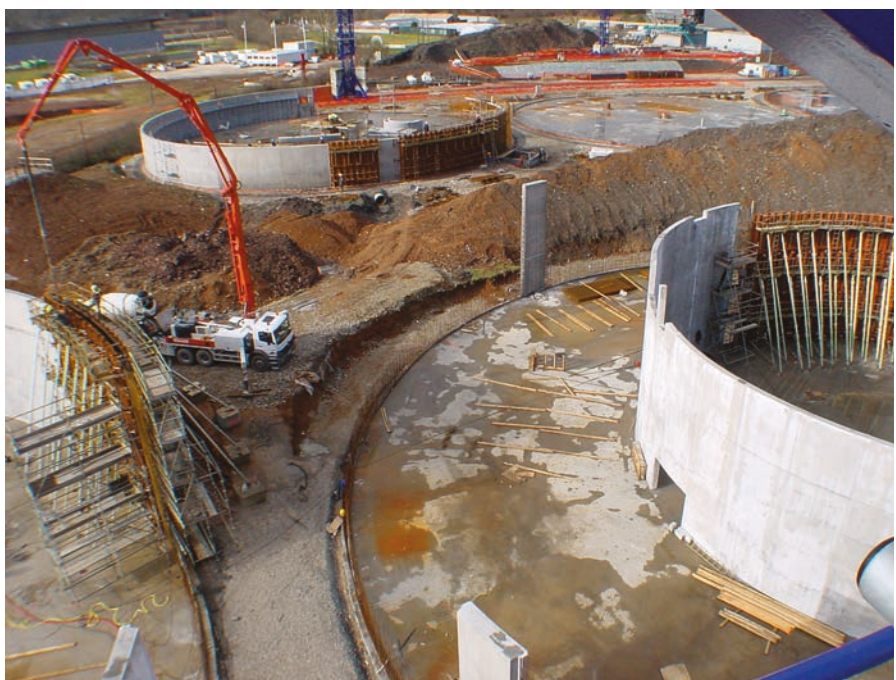
Waste water treatment plant, F-Brive la Gaillarde; Vigier/Sogea Sud Ouest, F-Toulouse
