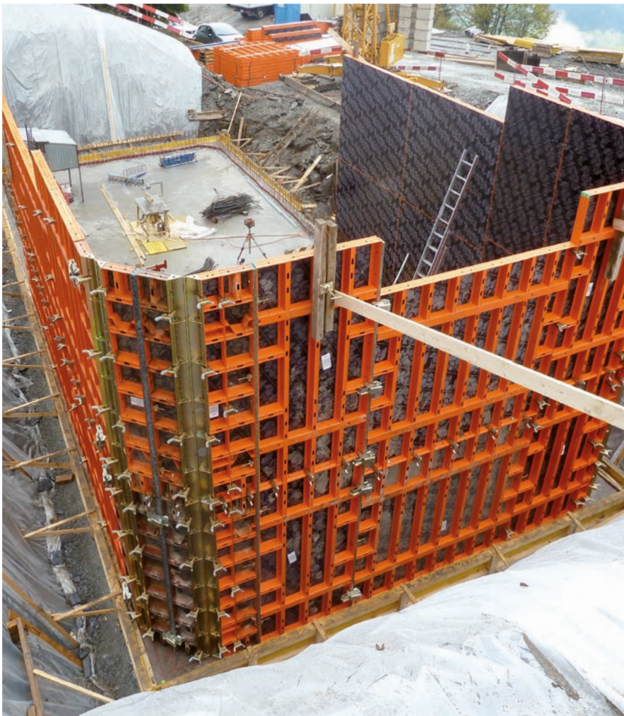
Water reservoir Surcuolm, CH-Obersaxen GR; Candrian SA, CH-Illanz
