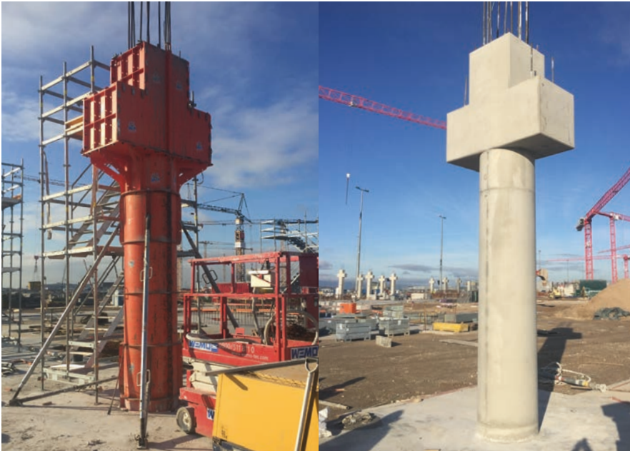
Construction of new terminal, Frankfurt Airport; Adolf Lupp GmbH & Co. KG AV/BL
