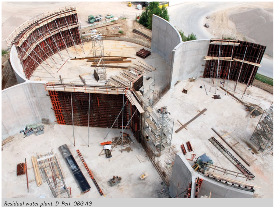
Residual water plant, D-Perl; OBG AG
