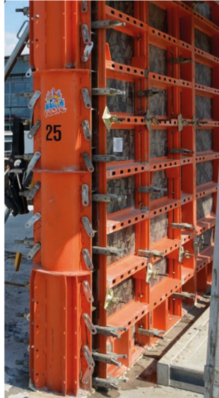
Semi-circular end of a wall in a sewage plant, built by combining circular column half circles with the Athlete formwork.
