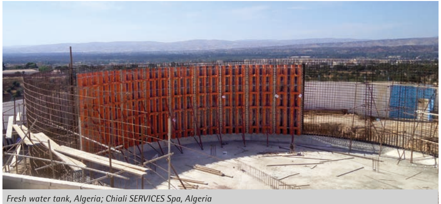
Fresh water tank, Algeria; Chiali SERVICES Spa, Algeria
