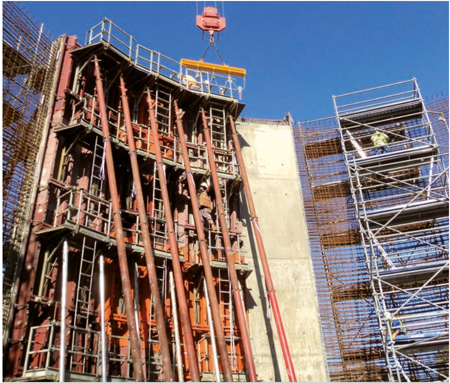
Waste water treatment plant, F-Brive la Gaillarde; Vigier/Sogea Sud Ouest, F-Toulouse
