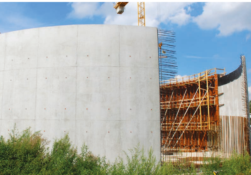
Biogas plant, D-Bürstadt; Wilms, D-Bürstadt
