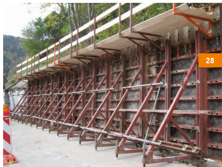
Retaining wall, renovation of the Thale through road; Umwelttechnik & Wasserbau GmbH, D-Blankenburg/Harz
