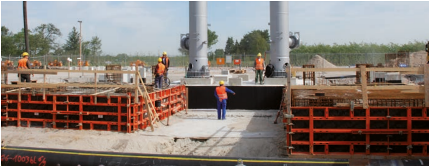
Natural gas storage stations, D-Etzel; Knoll GmbH, D-Haren
