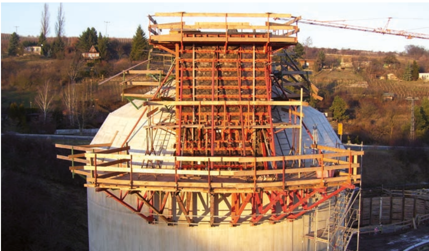
Round pinnacle of sewage treatment plant digestion tower, D- Rollsdorf; beton & rohrbau GmbH & Co.KG, D-Halle
