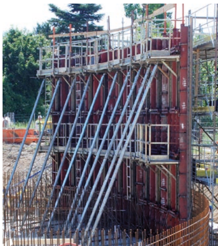
Drinking water treatment plant Montry, F-Montry ; Gagneraud Construction, F-Sarcelles
