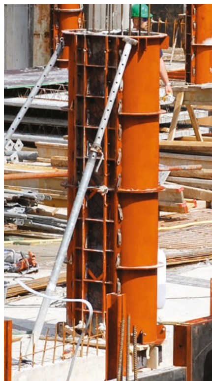
In these oval columns, special panels with steel face were connected directly to the half circles of the circular column formwork.
