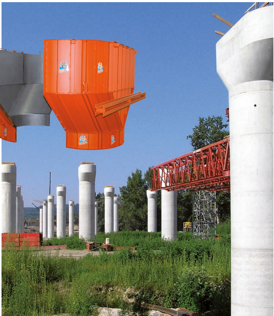
Bridge pier Danube bridge Traismauer, Link Nord RFB; Co. Alpine Bau GmbH, A-Vienna
