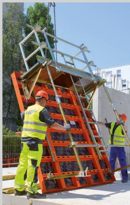
After pre-assembly or unfolding the platforms, the formwork is placed together with stages and props.
