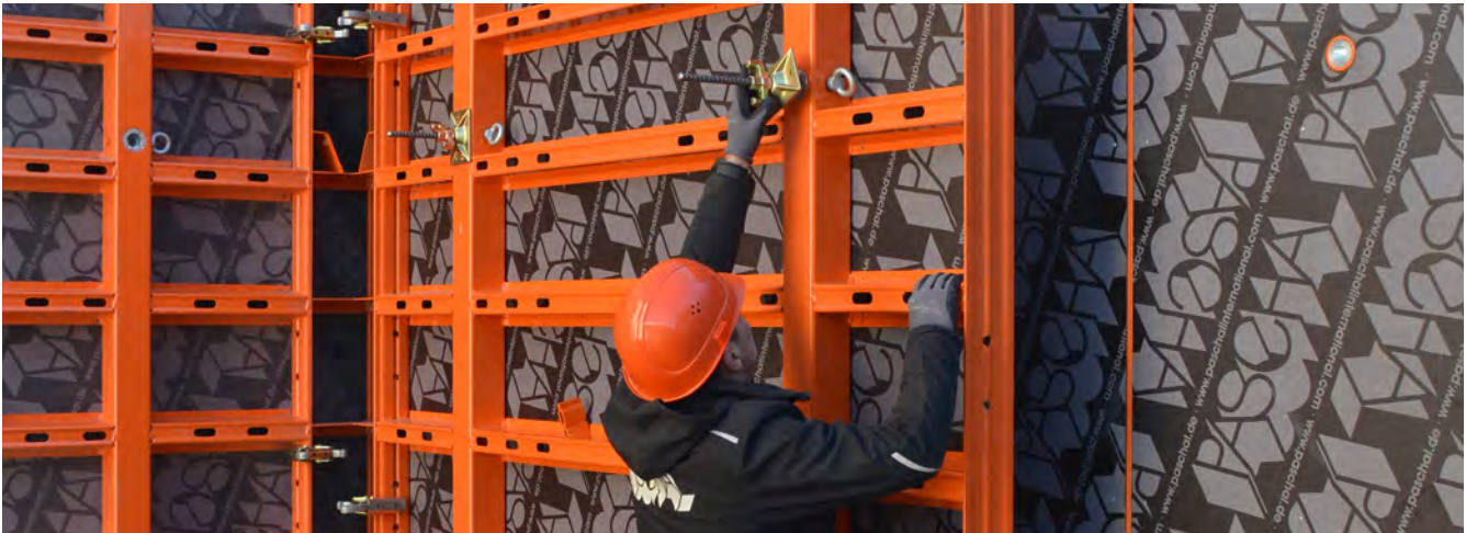
One-sided anchor technology makes the formwork anchors easy to operate by just one person.
